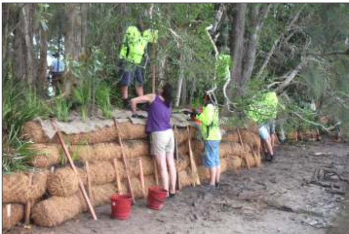
CCCG volunteers installing coir log walls on the banks of the lake in 2014
